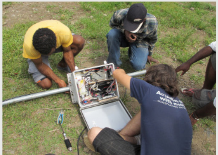
The VBTS team works to install a system in rural Papua. Unlike other telecommunications infrastructure, VBTS does not require multiple connections or expensive equipment.
